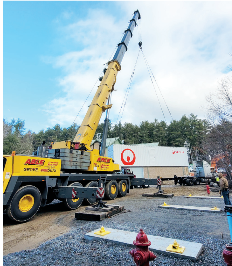
Major system components, including the trailers shown above that house the PFAS filter vessels, were delivered to the NAWTP on December 5, 2023. This facility began supplying water with non-detectable levels of PFAS to our distribution system on June 1, 2024, after nearly four years of effort on this project!
